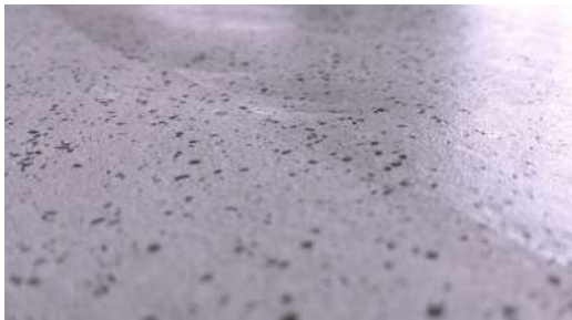
Left at the bottom: unprotected
