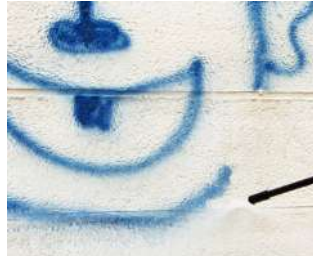
If the protected surface is soiled with graffiti: clean surface with a high pressure cleaner. Then re-apply the PROWALL II onto the cleaned areas.
